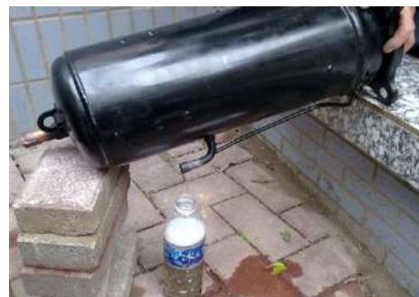
Figure 6-2.5: Draining oil from a compressor
